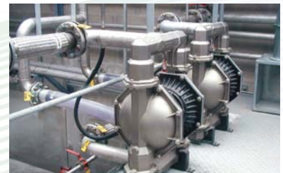
3" stainless steel diaphragm pumps installed on a bulk transfer process
