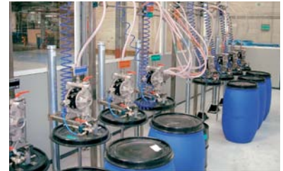
1/2" diaphragm pumps installed in a colouring process
