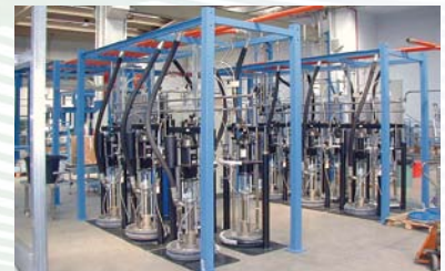
Large extrusion piston pumps, 13:1 ratio, installed on an offset ink formulation system process
