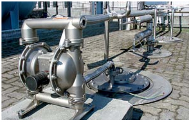
1 1/2" diaphragm pump installed in a chemical process to transfer chloride methylene
