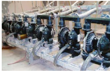
3" diaphragm pumps mounted on a skid to transfer clay in a ceramic manufacture
