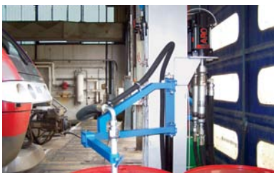
2-ball piston pumps 9:1 ratio, used in a customised lubrication process
